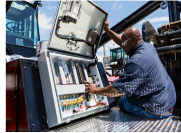
Easy Access to Heavy Duty Circuit Breaker Panel & Breaker Reset Switches
