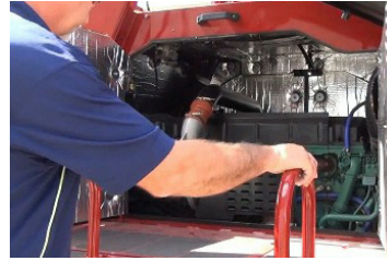
Service & Inspections from Running Board Large Bay Doors Provide Full Access
